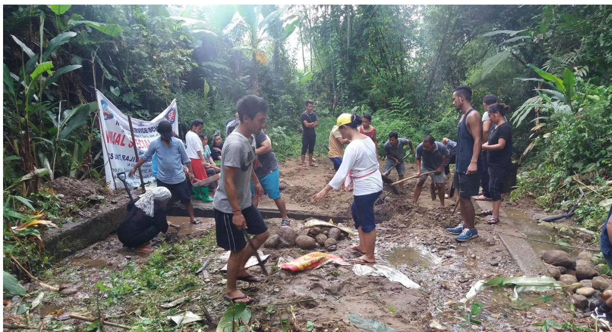
Watershed Management: Clearing debris of the Intake Point of Water Source by the NSS Volunteers, POs and Villagers at Lekha Village
